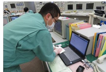
*In the main control room of the power plant, common equipment is disinfected with alcohol twice a day.
