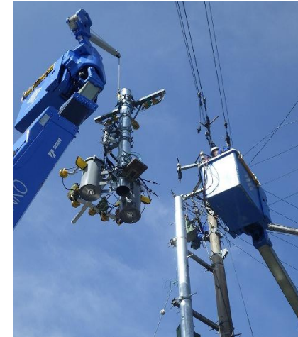
Prefab construction method makes pole-top work more efficient by pre-assembling equipment before installation (Yondenko)
